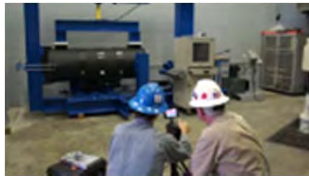
24" STEAM LINE SUPPORTS
