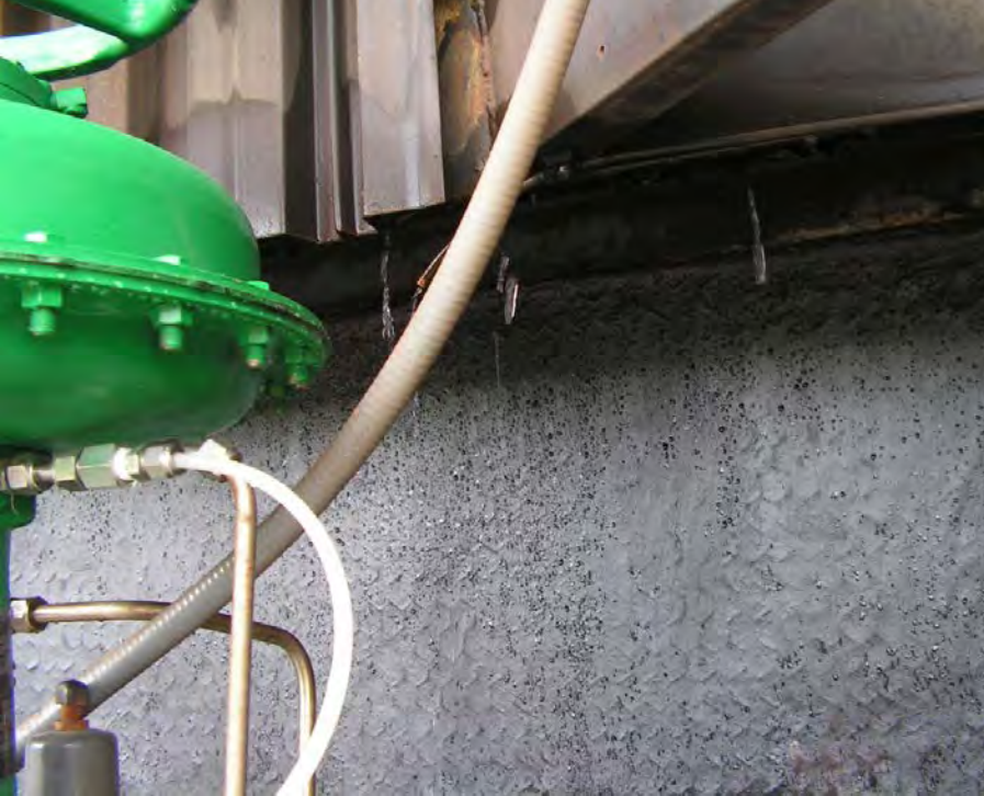
RAIN WATER LEAKING FROM BOTTOM OF PENTHOUSE
