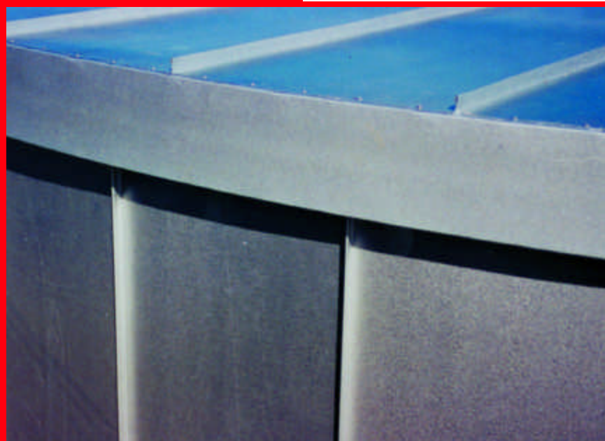
60' diameter x 40' high storage tank insulated with 1 1/2" thick PIR on the walls and 3" thick mineral wool on the roof. Photo courtesy of Associated Insulation.
