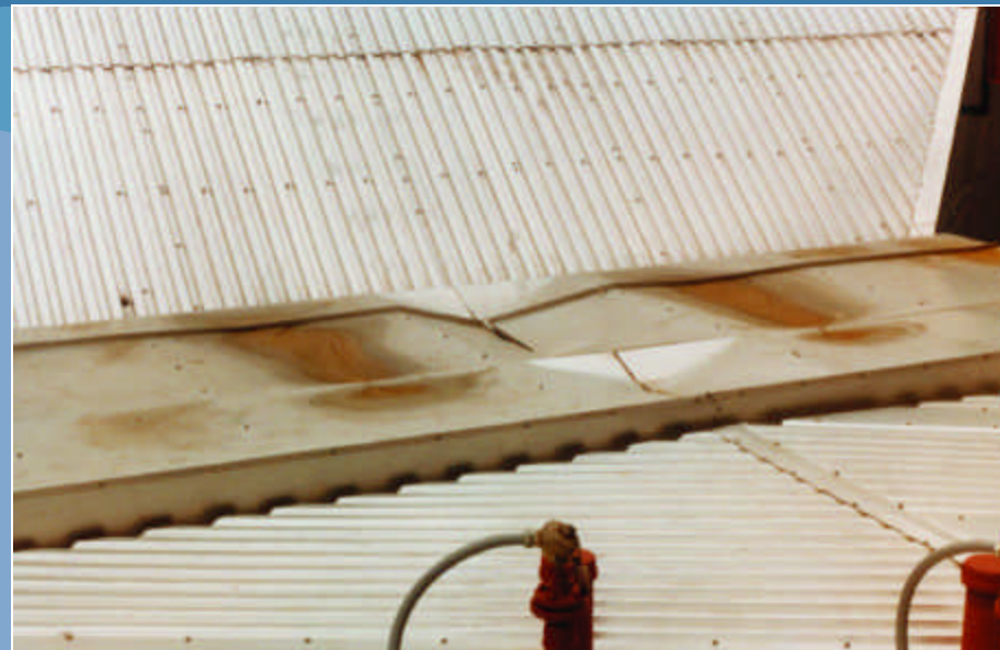
A poorly designed and/or installed lagging and insulation system with ponding.
