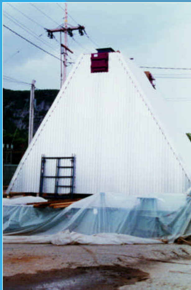
Precipitator hopper completely insulated and lagged.
