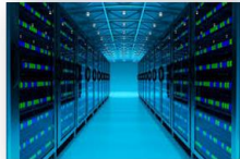
Communications/ Data Centers
